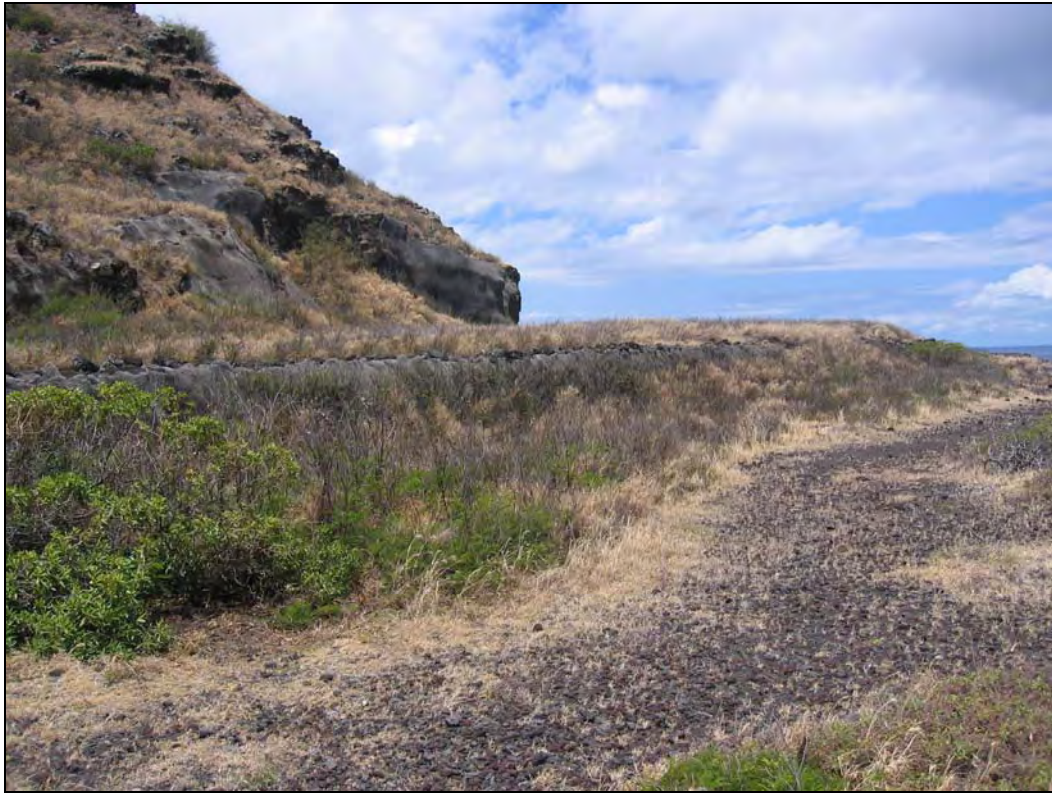
Fig. 33: Edge of Terraced, Cut and Fill Road Bed Stabilized with Pressure-Spray Gunite (Facing Southeast).
