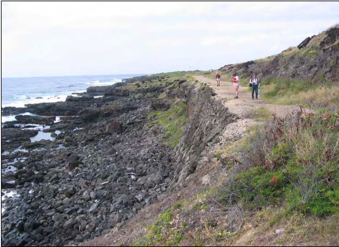
Fig. 21: Rock-Faced Retaining Wall for Railway Bed Southeast of the Project Area (Facing Northwest)
