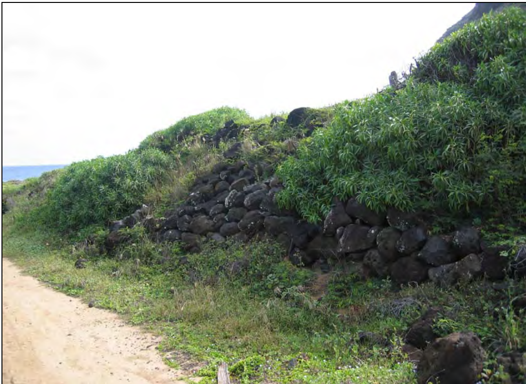
Fig. 26: Rock Retaining Wall along Mauka Edge of Railway Bed near Northern Bend in the Alignment (Facing Northwest). Note use of water-worn stones.
