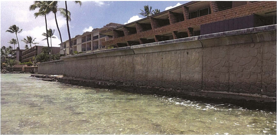
Figure 5 - Central portion of the seawall with exposed footing, May, 2020.
