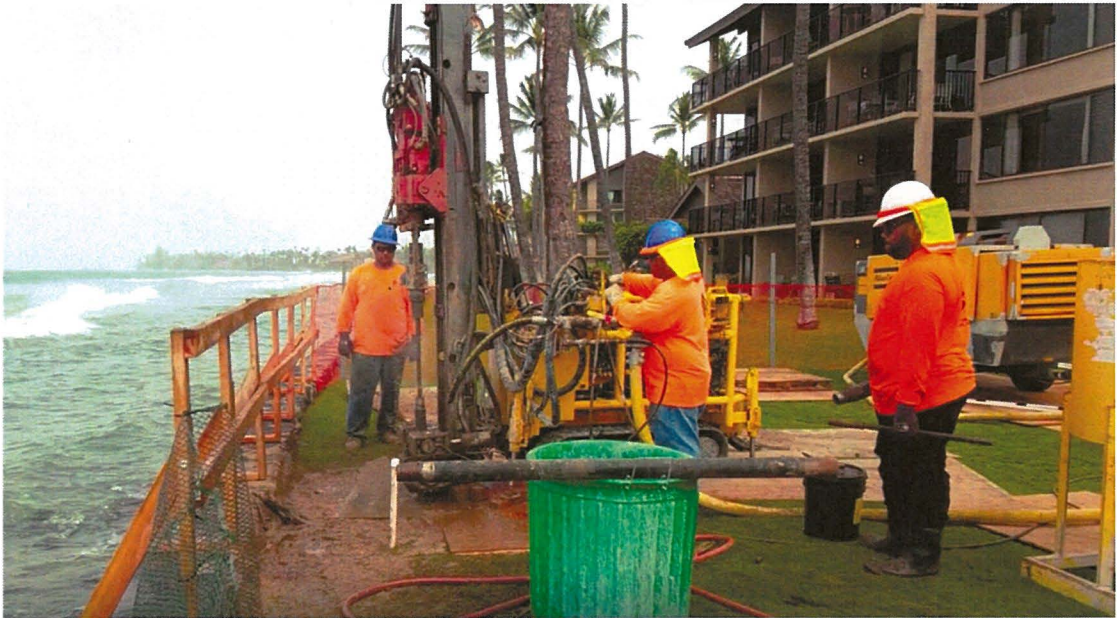
Figure 8 - County approved injection grouting to repair the seawall at the nearby Papakaea Condominium in 2015.
