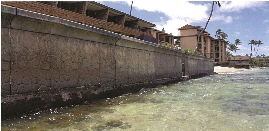
Figure 7 - Southern portion of the seawall with footing exposed, May, 2020.
