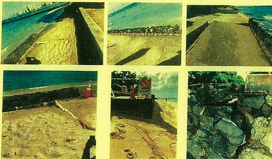
Figure 1 – Damaged Section of Ramp and Seawall, Provided by Applicant
