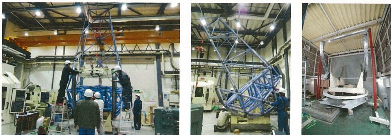
Figure 4. The mechanical truss structure that supports the telescope and the rotation table are being completed in Japan.
