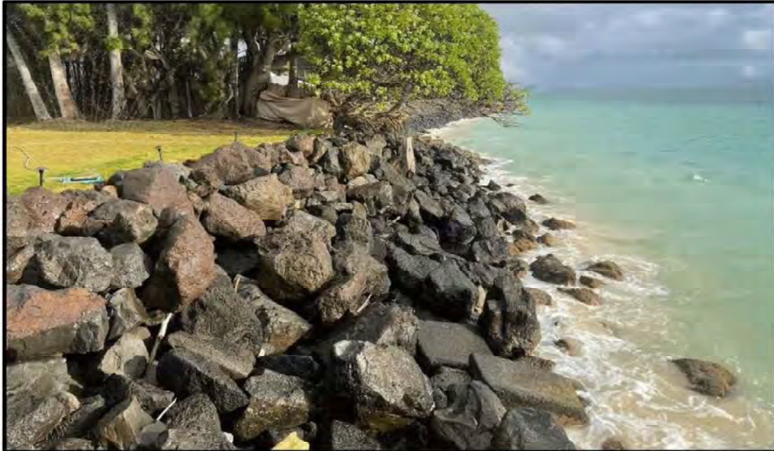
Note: Photo of revetment looking north. Waves are washing up the revetment.
