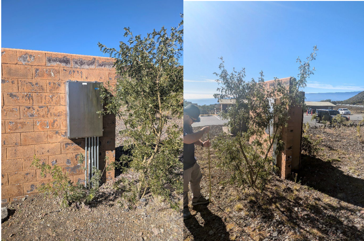
Figures D and E, showing māmane near the rear breaker box of the electrical panel. CMS will attempt to relocate the smaller māmane directly in front of the breaker box and will prune the larger māmane.
