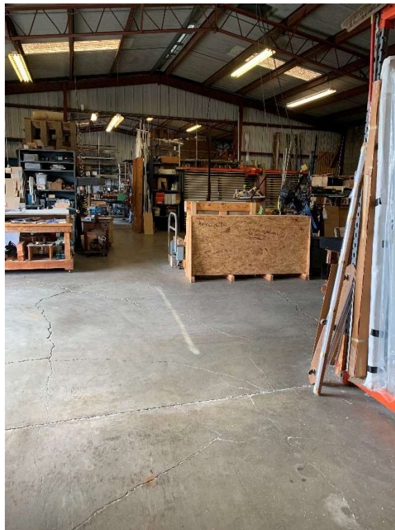
VIEW OF BACK OF ORIGINAL WAREHOUSE. NOTE STRESS CRACKS IN FLOOR. WALL IN BACKGROUND IS END OF ORIGINAL WAREHOUSE
