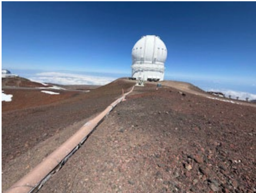
Fig 2. The aboveground conduit, insulating cover, and small concrete anchors span a distance of roughly 270 feet between the CFHT weather tower and Gemini North.
