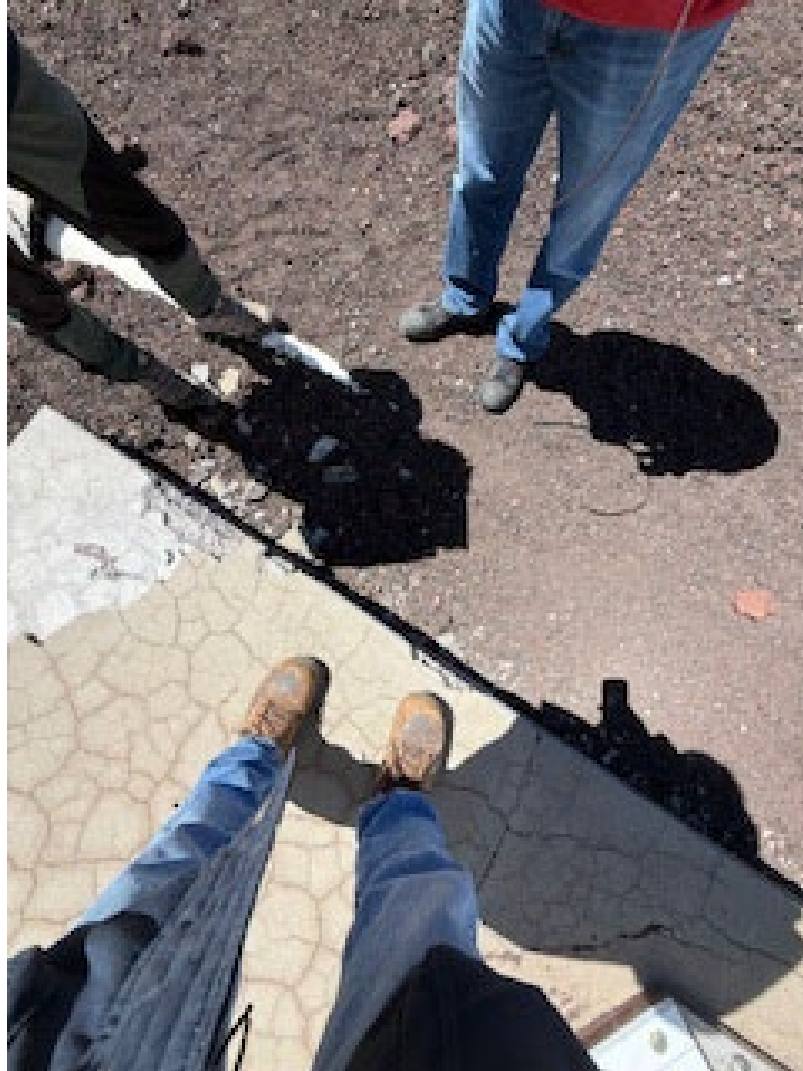
Fig 3. The conduit transitions underground at the edge of the weather tower concrete pad, denoted by person to left of image, with foot on conduit
