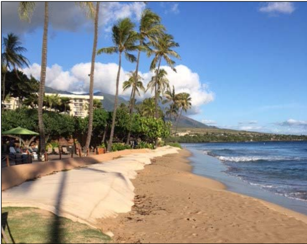
Figure 3-4 Erosion protection skirt (Kaanapali, Maui, Hawaii)
