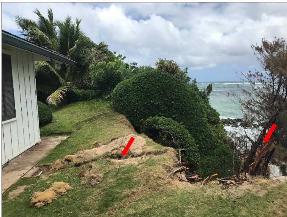
Figure 14 Collapsed trees and damaged water infrastructure, TMK (1) 5-5-002:019
