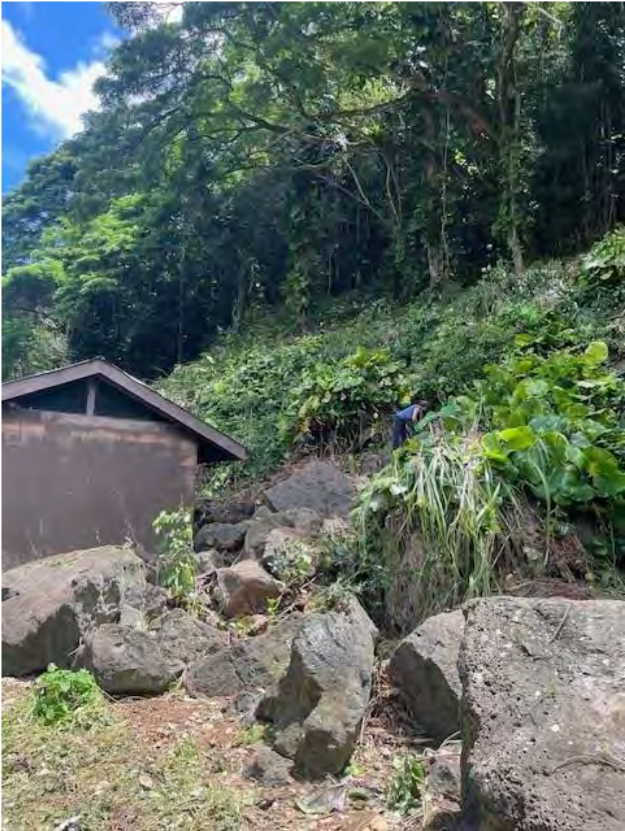
Photo 3. Facing northwest at the rockfall mitigation location behind the Community Resource Center
